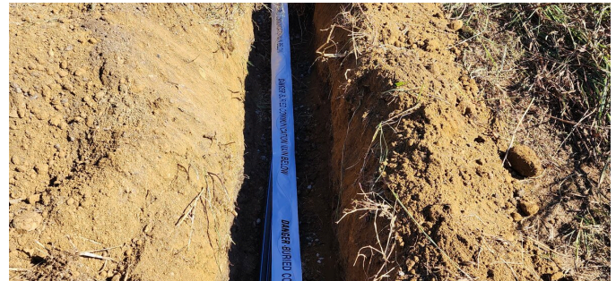
Conduit run from the station to the orifice
