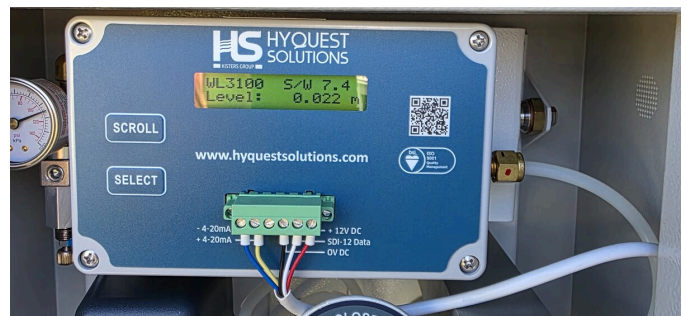
Bubbler unit checked and purged
