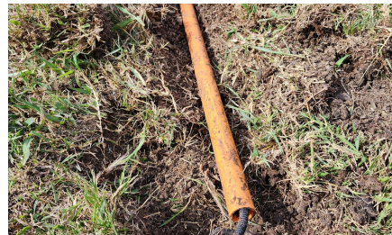
Cable run in conduit to the pit
