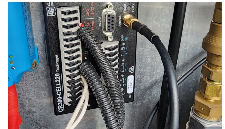
Probe wired into the station logger
